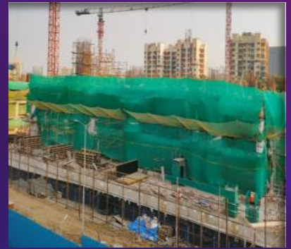
Green net duct control
